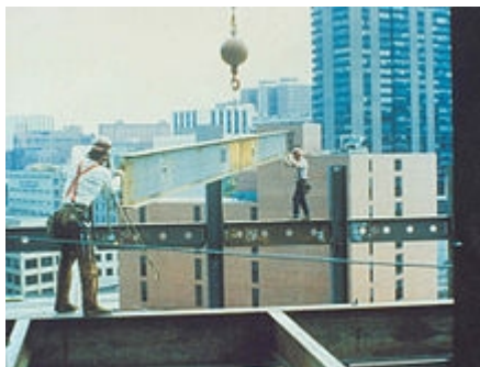
At-risk workers without appropriate safety equipment
